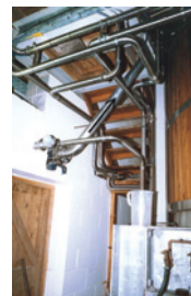
Grist case / miller outlet below mash tun, seepex pump transporting mixed grain and hot water back up into mash tun
