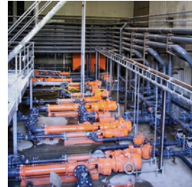
seepex pumps in the central fodder kitchen during the distribution of the fodder pulp from the mixing containers in various pipes
