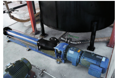
Halar coated seepex pump underneath storage tank.
