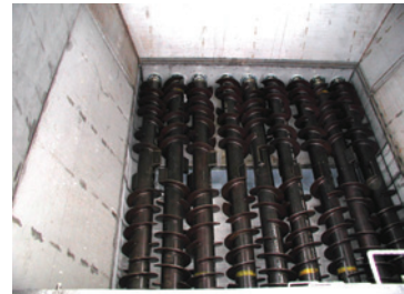
Live bottom reception silo with 9 bi-directional screws
