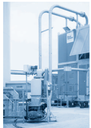
Two manually adjustable seepex pumps BTI 10-24 with bridge breaker, Product: dewatered primary sludges from belt presses, 25% ds, Application data: 1.0 - 2.0 m 3 /h, 24 bar, discharge into dryer, Pressure pipe: 6 m horizontal, 9 m vertical, Ø 200 mm, Accessories: additional extension hopper
