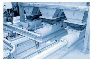
Application data: 1.0 - 1.8 m 3 /h and 0.2 - 0.7 m 3 /h, 10 bar, discharge into dryer, Pressure pipe: 10.5 m horizontal, 9.5 m vertical, Ø 250 mm
